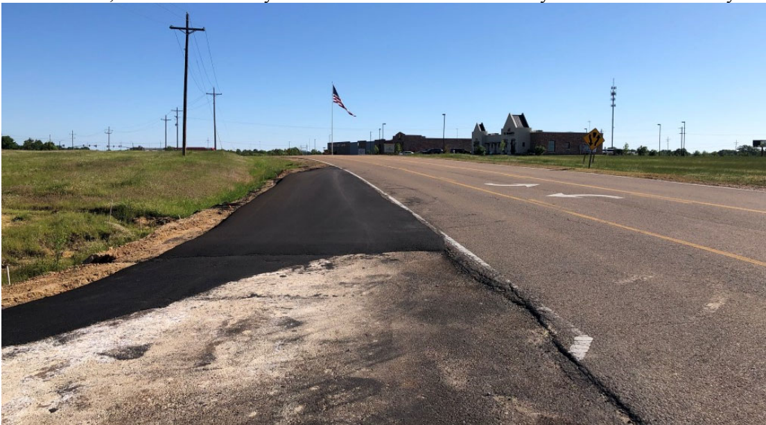
Looking north on 3-Lane Calhoun Station Parkway from Gluckstadt Way near Calloway’s
