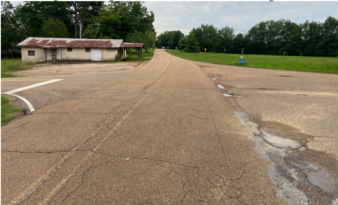
Below: Looking south on Livingston Vernon Road at Stokes Road/abandoned gas station.
